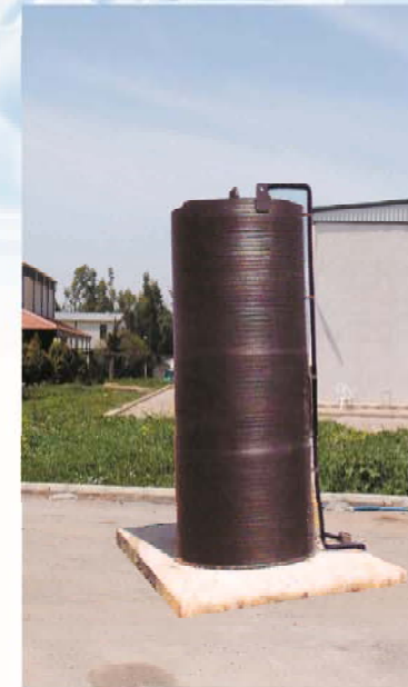
Chemical Storage Tank
