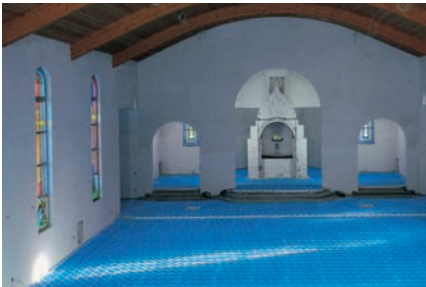
Surface regulation systems featuring Hewing PE-Xc pipes are used in a variety of locations, such as churches, for example ...
